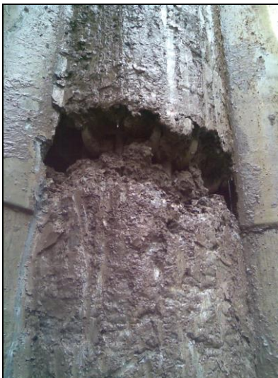
A defective pile
